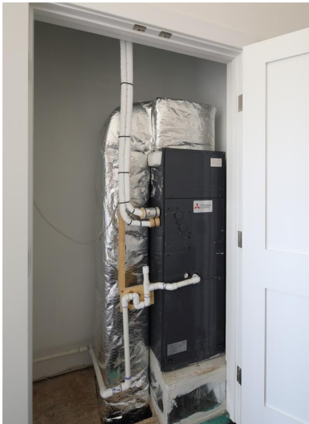
The Bridgeport Properties townhomes feature high-efficiency HVAC.
