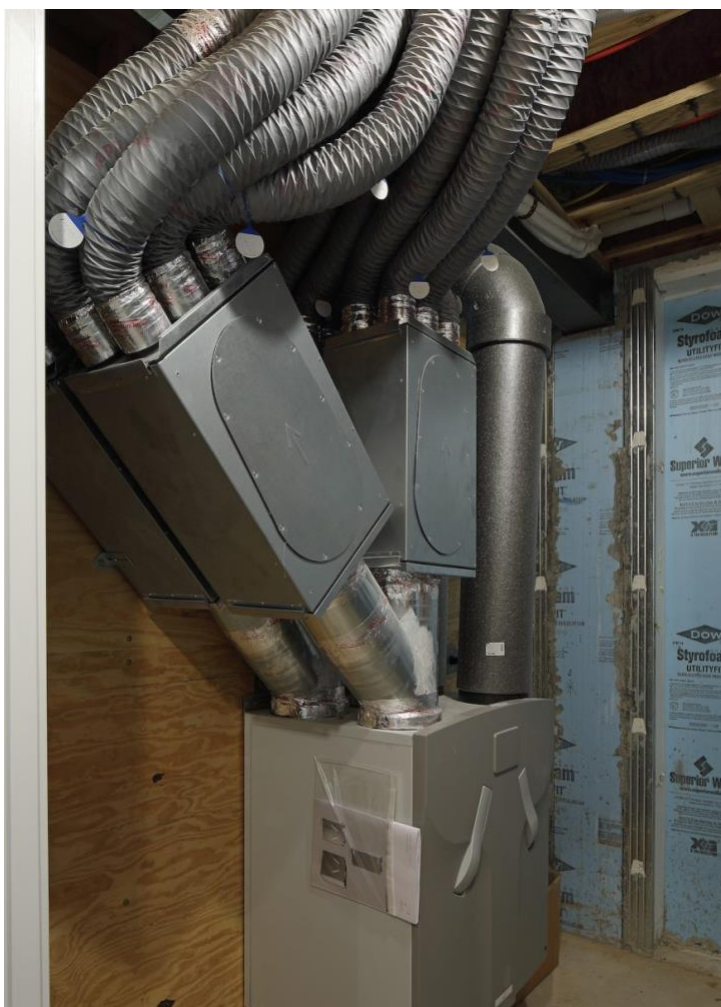
The energy recovering ventilation system in the Bridgeport Properties townhomes.
