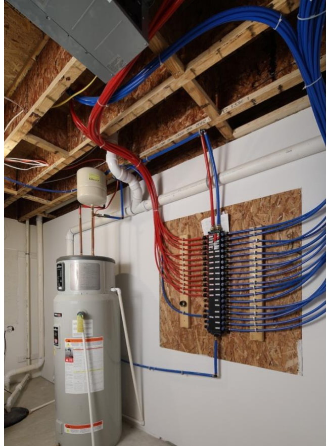
A sophisticated manifold saves both water and energy. Construction photos courtesy of Alter Eco, LLC.
